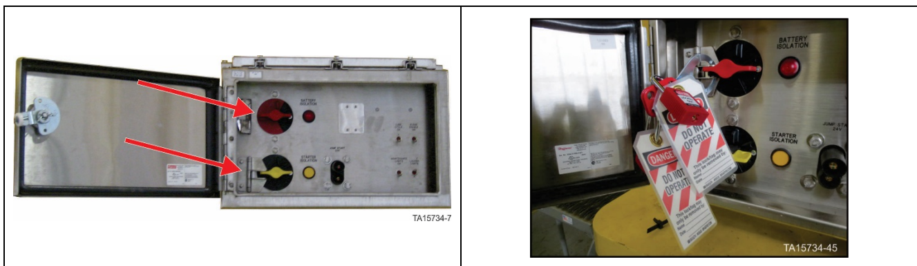
Figure 8. GEN 2 Battery Isolation Box – Battery isolation switch in OFF position with locks in place
