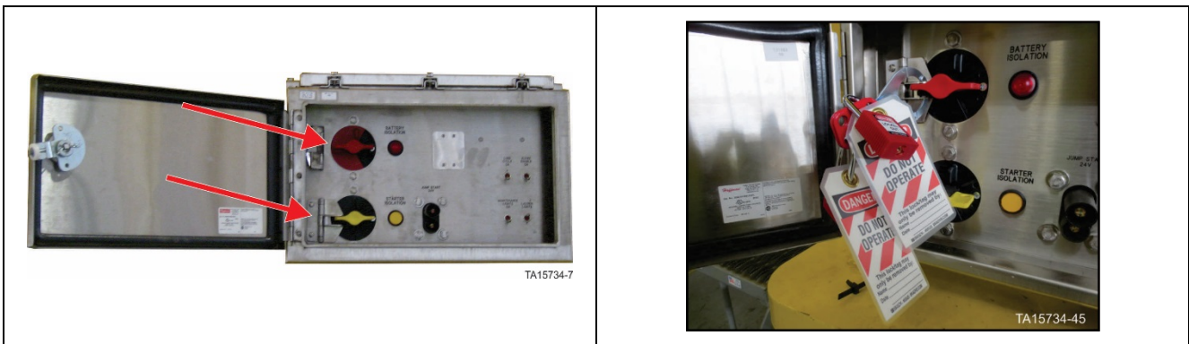
Figure 12. GEN 2 Battery Isolation Box – Battery isolation switch in OFF position with locks in place
