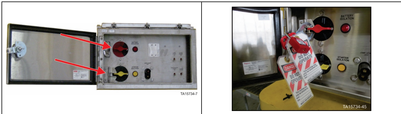
Figure 23. GEN 2 Battery Isolation Box – Battery isolation switch in OFF position with locks in place
